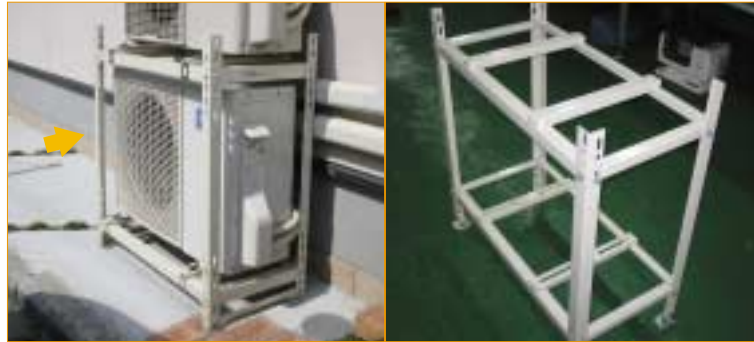
Trestle for outdoor unit of air conditioner (Painted)
