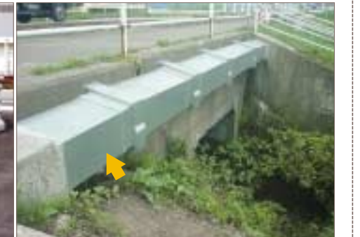
Fireproof protection for optical fiber
