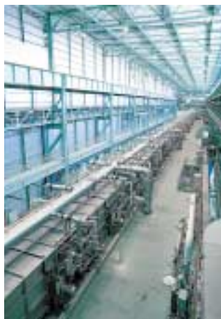
② HCGL annealing furnace (horizontal radiant tube furnace)
