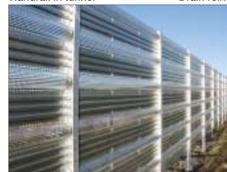
Snow barrier panel
