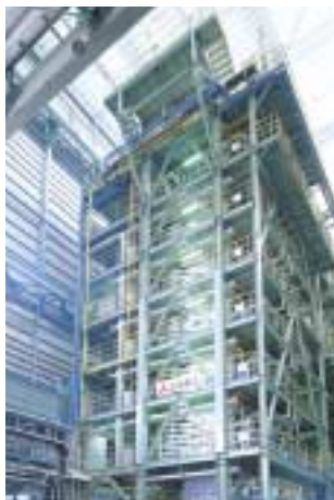
① HCGL annealing furnace (upright direct-fired reducing furnace)
