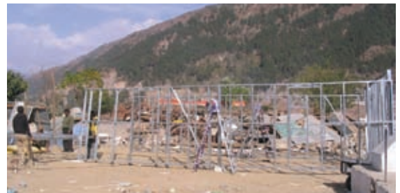
The house used in the tests measured approximately 2.6 x 2.8m in plan and 2.4m in height, with a brick veneer cladding and plasterboard interior lining. A roof slab weighing 1,500kg was placed on top and was supported by the steel frame to simulate the equivalent mass of a house roof in a typical full-scale single storey brick home.
