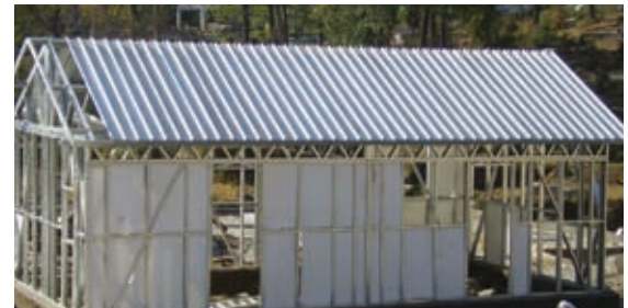
In countries subject to seismic activity, building design, engineering and construction must be specifically tailored to withstand those unique environmental hazards and I think the world is teaching us about that, -FRAMECAD Design Services Manager, Dr Darrin Bell.
